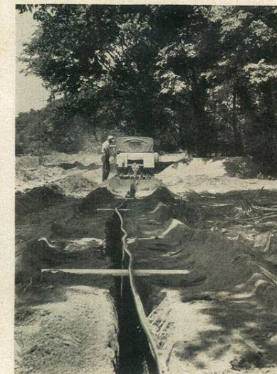
GROUND PIPE for heat pump is laid in deep trench dug by jeep-drawn ditch digger. Pipe is buried below frost line where year-round temperature remains nearly constant. Here in Jeffersonville, Indiana this temperature is about 52°F.
