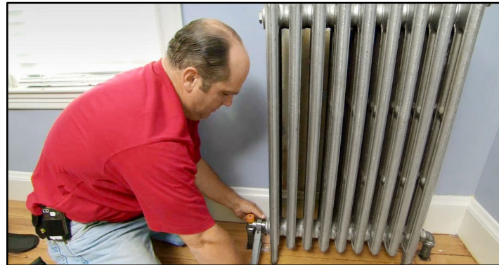
Hot Water Radiators (160°F – 180°F)
