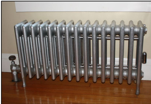
Steam Radiators (212°F+)
