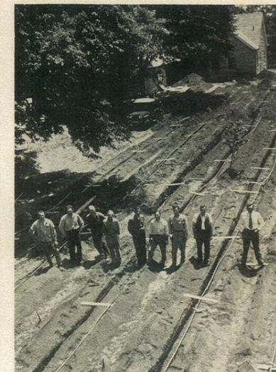
PIPE TRENCHES cover whole lawn in this heat pump installation. Men are the crew necessary to install the Miracula. Miracula can also get source of heat from pipes to wells, lakes or streams, and in warm areas from the air itself.
