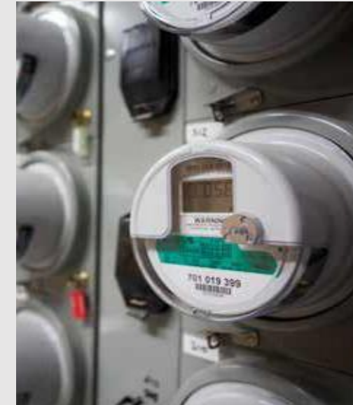
Electric Metering from Financing High-Performance, 2020
